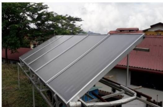
Fig. 2. The active Solar Water Heating system installed at CST
