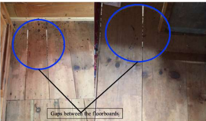
Fig. 6. Spaces Between the Floorboards at Changdatang (Timber)
